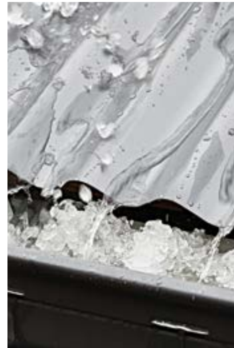
Accumulated hail in a gutter without gutter mesh installed
